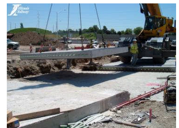
Crews install a pre-cast slab on the I-88 loop ramp at the IL 83 Interchange
