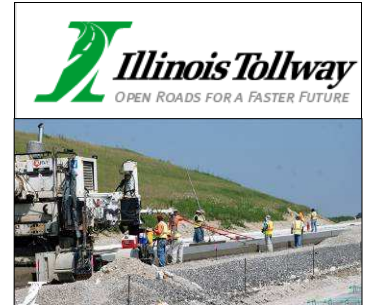
Crews follow the paving train to smooth out the new concrete on the southbound lanes of the South Extension near 127th Street.
