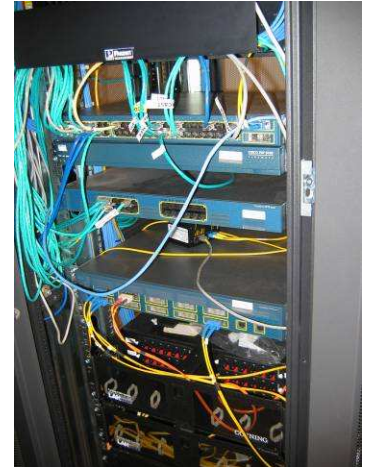
Connectivity is the key at the Lake County Illinois Traffic Management Center
